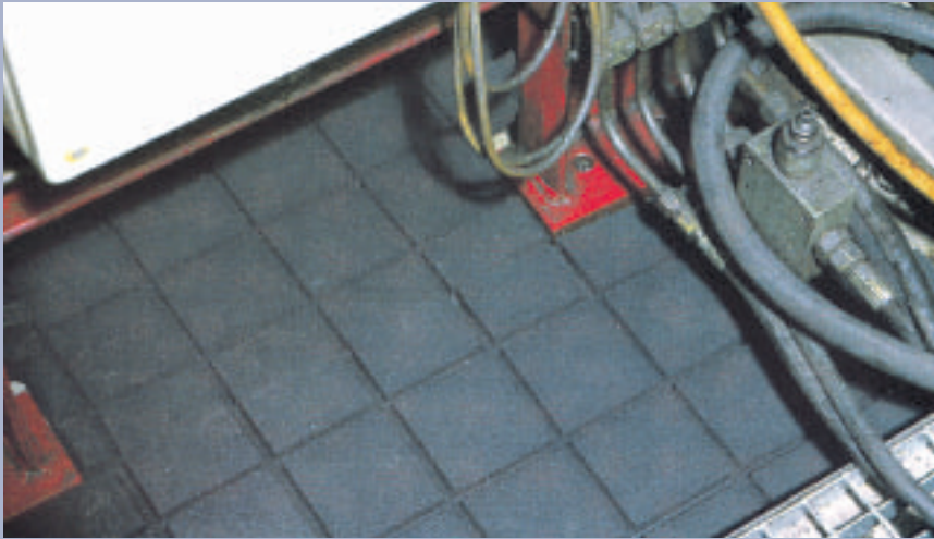
Protection of hydraulic machines
